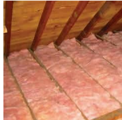
Figure 15 - Adding ceiling insulation in older buildings is one of the most cost effective methods of saving energy.
