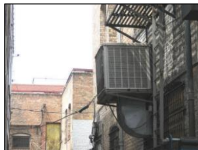
Figure 168 - Heating and cooling units should be located at rear elevations such as shown here or on rooftop areas not visible from the street
