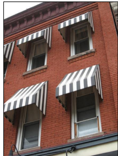
Figure 121 - Fixed awnings on upper floor windows at 623 Bloomfield Avenue enhance the energy efficiency of the building.
