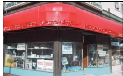
Figure 153 - NO - Do not allow signs to conceal or obscure historic building designs or detailing, such as an awning covering a historic transom.
