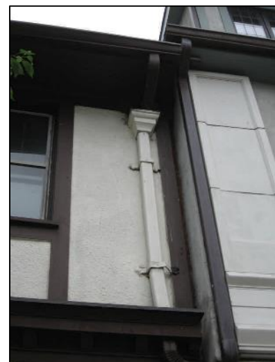
Figure 138 - This downspout at 620 Valley Road is recessed from the main façade, helping to conceal it. It is also painted the same color as the body of the building which decreases its visibility.
