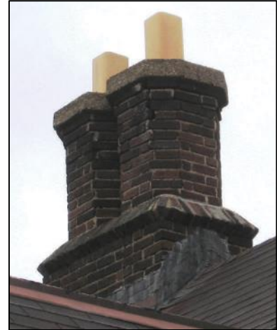
Figure 136 - Maintain and preserve original chimneys, like this distinctive octagonal pair at 45 Watchung Place.
