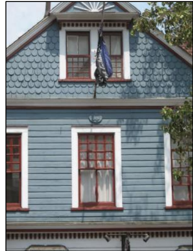
Figure 110 - Siding is unusual on commercial buildings. Where original siding exists, it should be preserved and maintained (411 Bloomfield Avenue).
