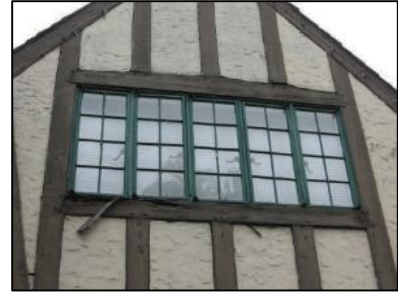
Figure 122 - Many of the Tudor Revival commercial buildings retain original wood or steel casement windows such as at 33 Watchung Plaza.
