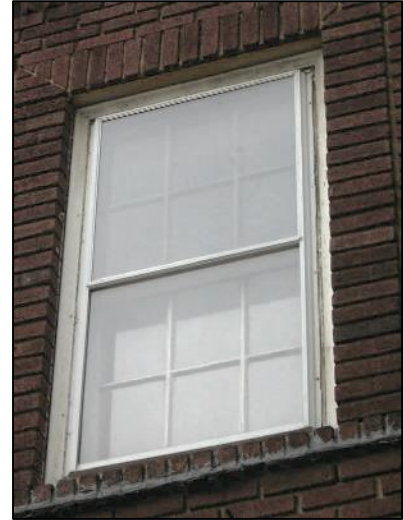
Figure 125 - The six-over-six wood sash window at 555 Bloomfield Avenue has an appropriate storm window
