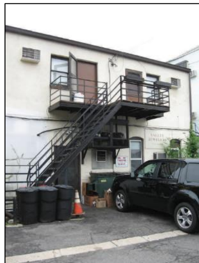
Figure 173 - Appropriately located rear façade fire escape at 219 Bellevue Avenue (above) and side elevation fire escape at 2323 Bellevue Avenue (below)
