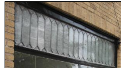
Figure 96 - Original transoms enhance historic character and are important elements of commercial storefronts (209 Glenridge Avenue).
