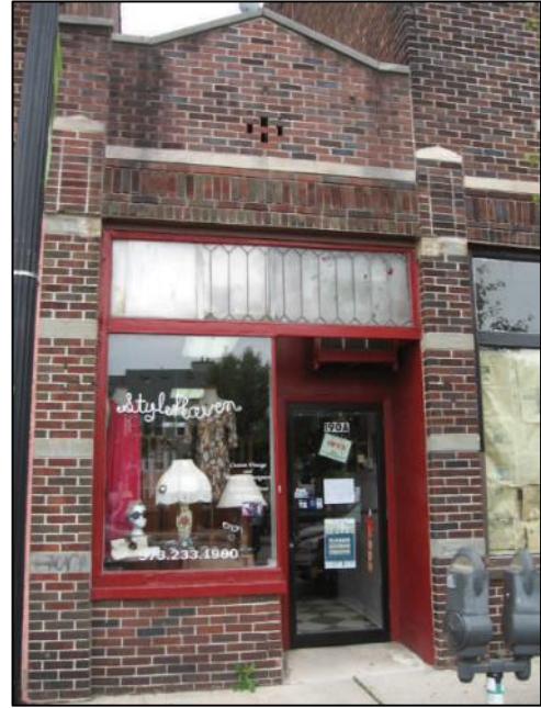
Figure 10 - The guidelines emphasize preservation of original features such as this storefront rather than removal or replacement (190A Bloomfield Avenue)
